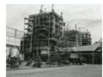
1968 Completed the first domestically produced 500 MW supercritical pressure boiler, Chubu Electric Power Chita Thermal Power Station Unit 3 (1,700 t/h)
