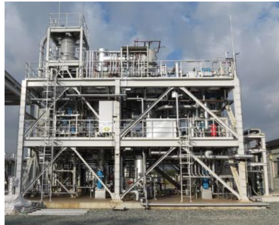
Biomass Gas Equipment
