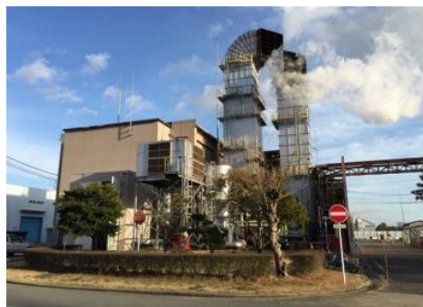
Takasago area facilities
