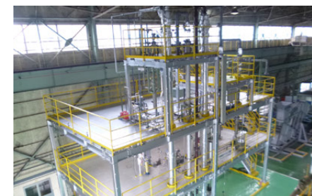
CO 2 recovery pilot equipment
