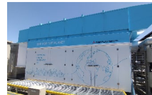
Hydrogen generator set for technical evaluation
