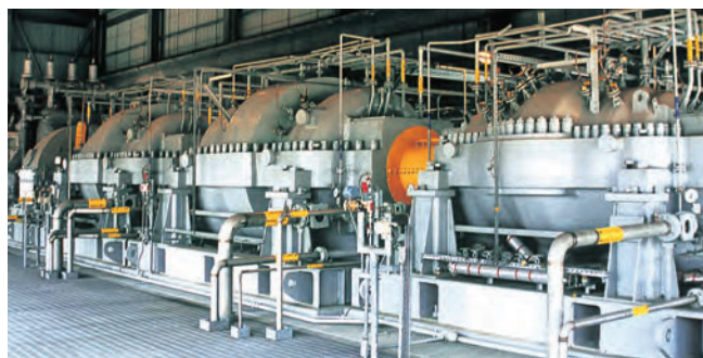
Cracked Gas Compressor & Steam Turbine for Ethylene
