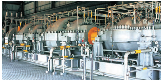
Cracked Gas Compressor & Steam Turbine for Ethylene
