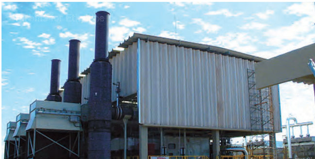
Gas Pipeline Station
