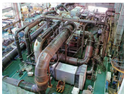
Integrally Geared Compressor for PTA Plant
