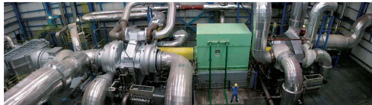
Air compressor (6-stage) and gas expander for PTA plant
