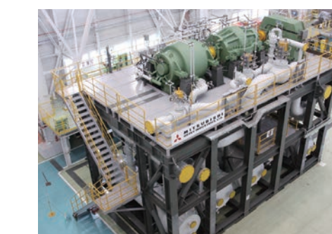
Nitrogen injection compressor module for ASU Plant
